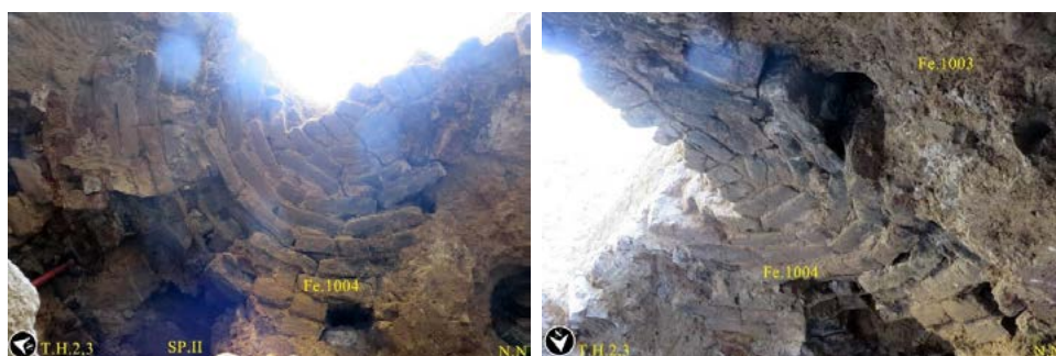
Fig. 15: Part of the brick dome or vault of the tomb and the vaulting technique in the Naqqārechi tomb (Janjan, 2022).
